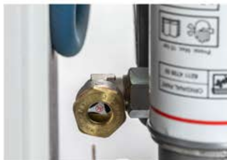
/// Oil level check
